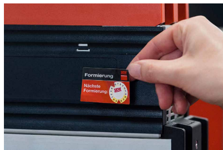
Labeling of checked frequency inverters
