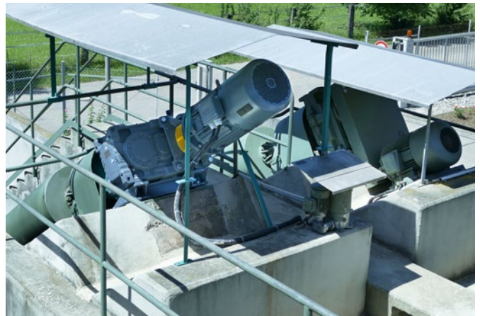
New drive with steel frame
