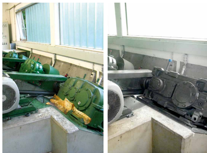
Left (before): bevel-helical gear unit (third-party drive) with belt drive
